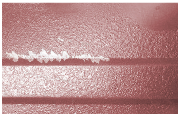
Note when scratched, the primer has been compromised as well as the presence of Zinc Oxide (white rust).
