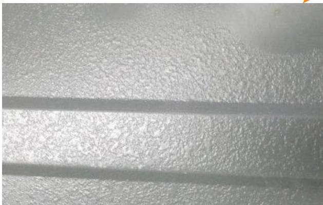
Close-up image of severe "Wet Stack Corrosion." Note smooth, normal surface in upper right corner.
